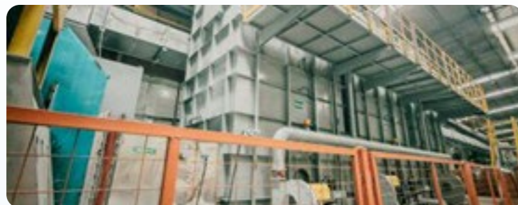
Regenerative Thermal Oxidizer Equipment
