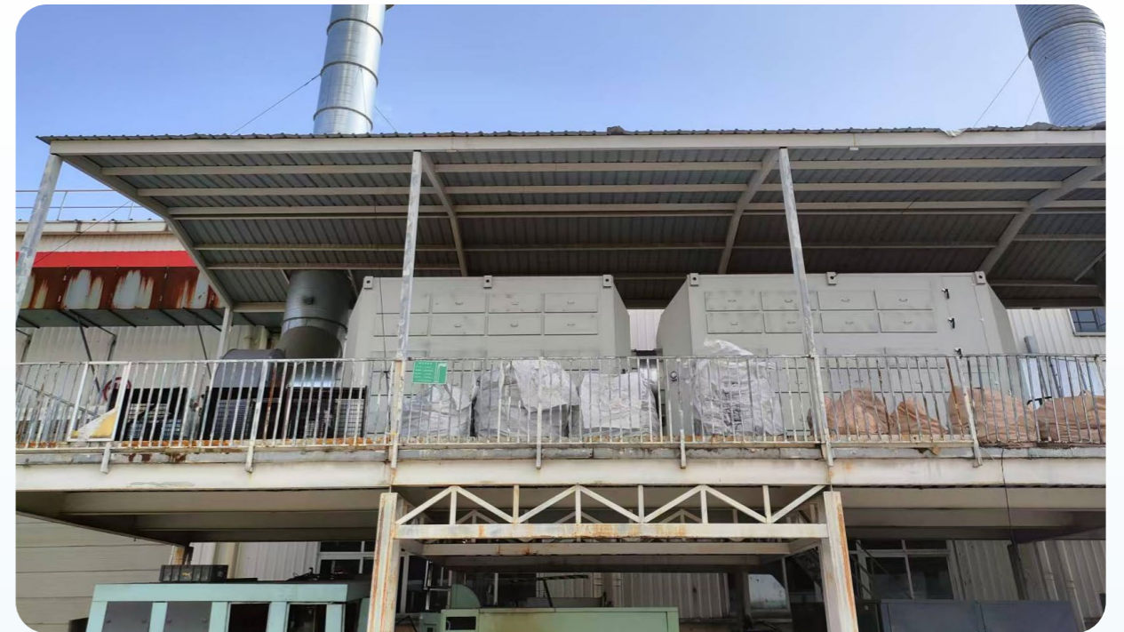
New Treatment Equipment of Waste Gas
